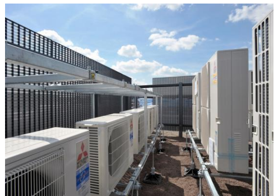
Mr. Slim (left) and Ecodan heat pumps on the roof
