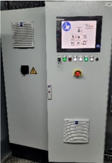
Pic 5: Control cabinet with Mitsubishi Electric GOT2000 HIMI
